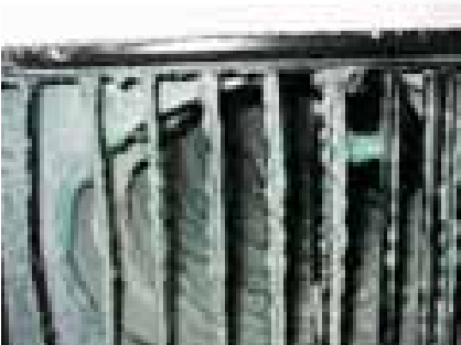
AHU 5-3 Return Air Grille, Before cleaning
